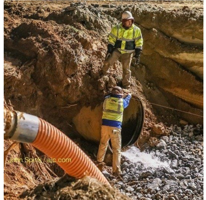
2018 Atlanta Water Main Break
